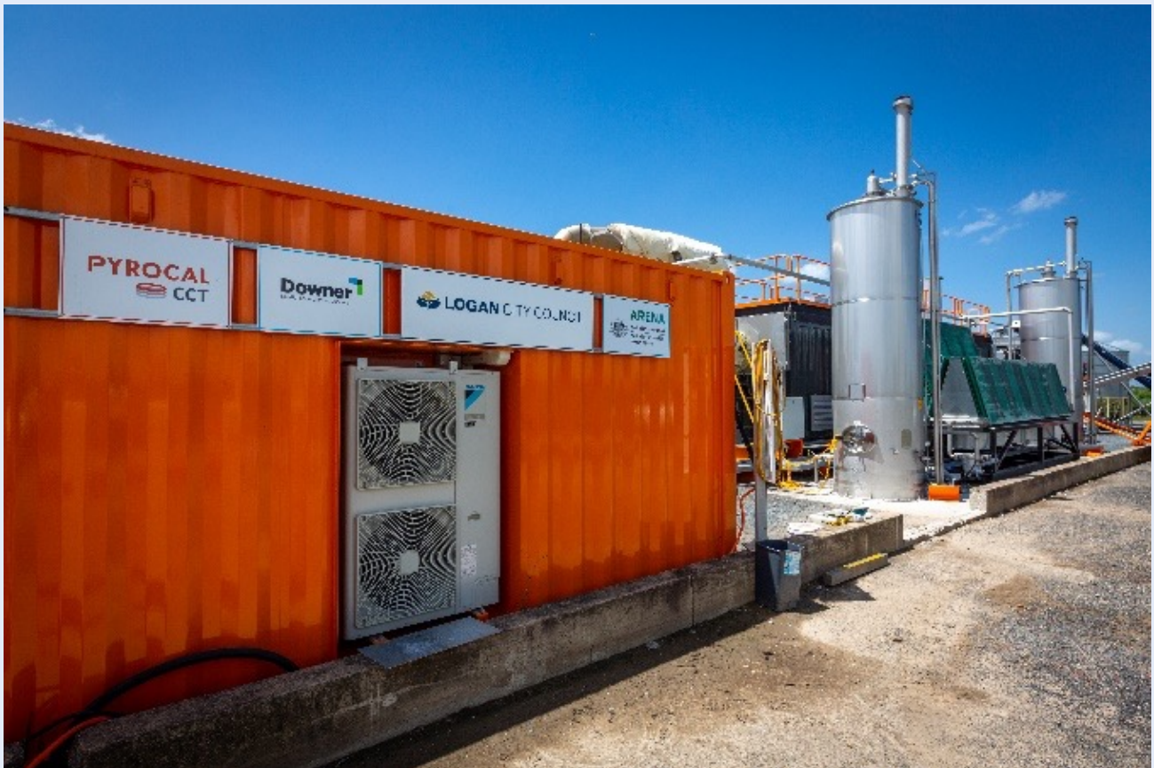
FIGURE 34 Loganholme WWTP gasification demonstration plant
