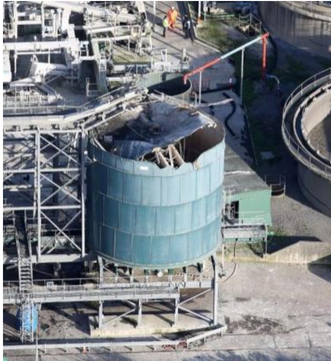
Figure 2-5: Ruptured silo at the facility showing the force of the explosion
