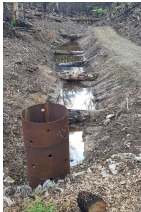
Debris racks and sediment dams (Melbourne Water).
