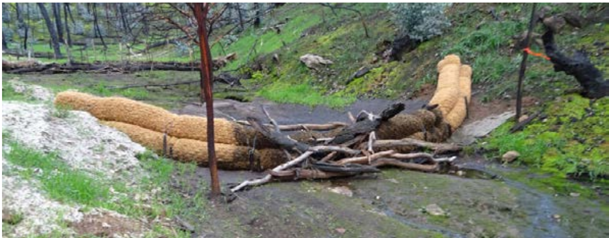
Coir logs with metal droppers – Millbrook Reservoir following the Sampson Flat Bushfire 2015 (SA Water)
